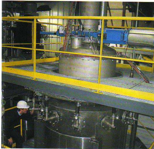
Xylowatt gasifier in the REGAL 300 kW cogeneration plant at Louvain la Neuve, Belgium (Details at www.xylowatt.com )
