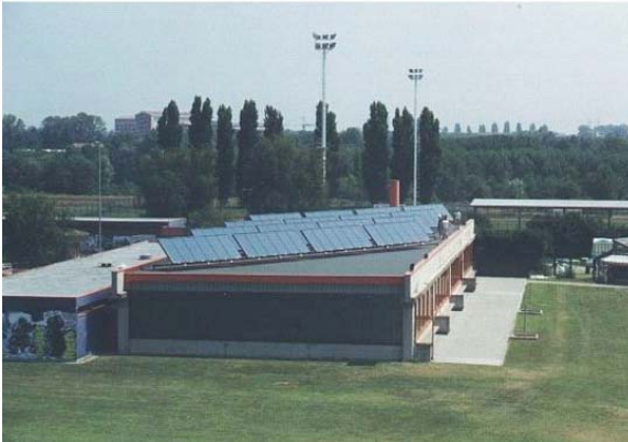
View of collectors filed at the municipal swimming pool of Melegnano (MI)
