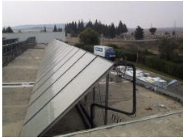
One collectors row in MEVGAL solar plant
